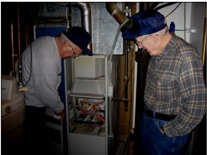
Haeg and Larson inspect a furnace.
